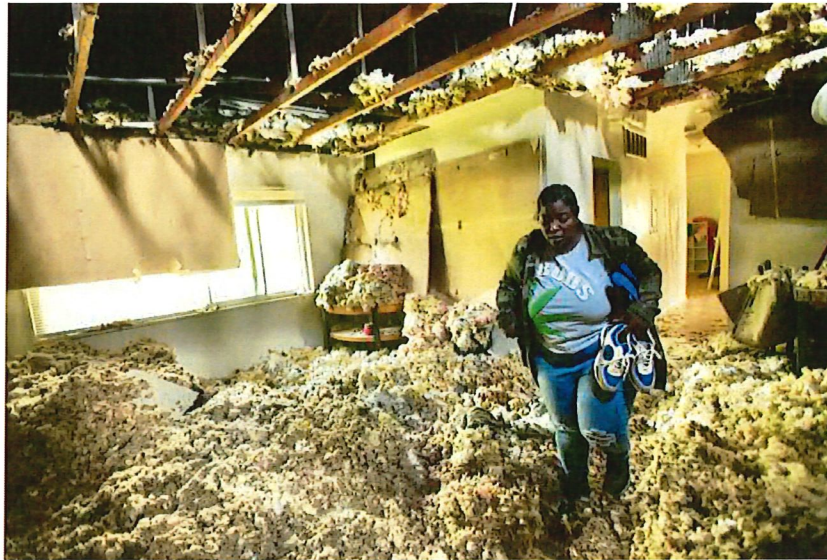
Demetrice Brown returns to her apartment to retrieve a few items after a fire ripped through the top-floor apartments in the 2900 block of Lakebrook Circle in Lansdowne early Sunday morning. Several families are displaced. (Amy Davis/Staff)
